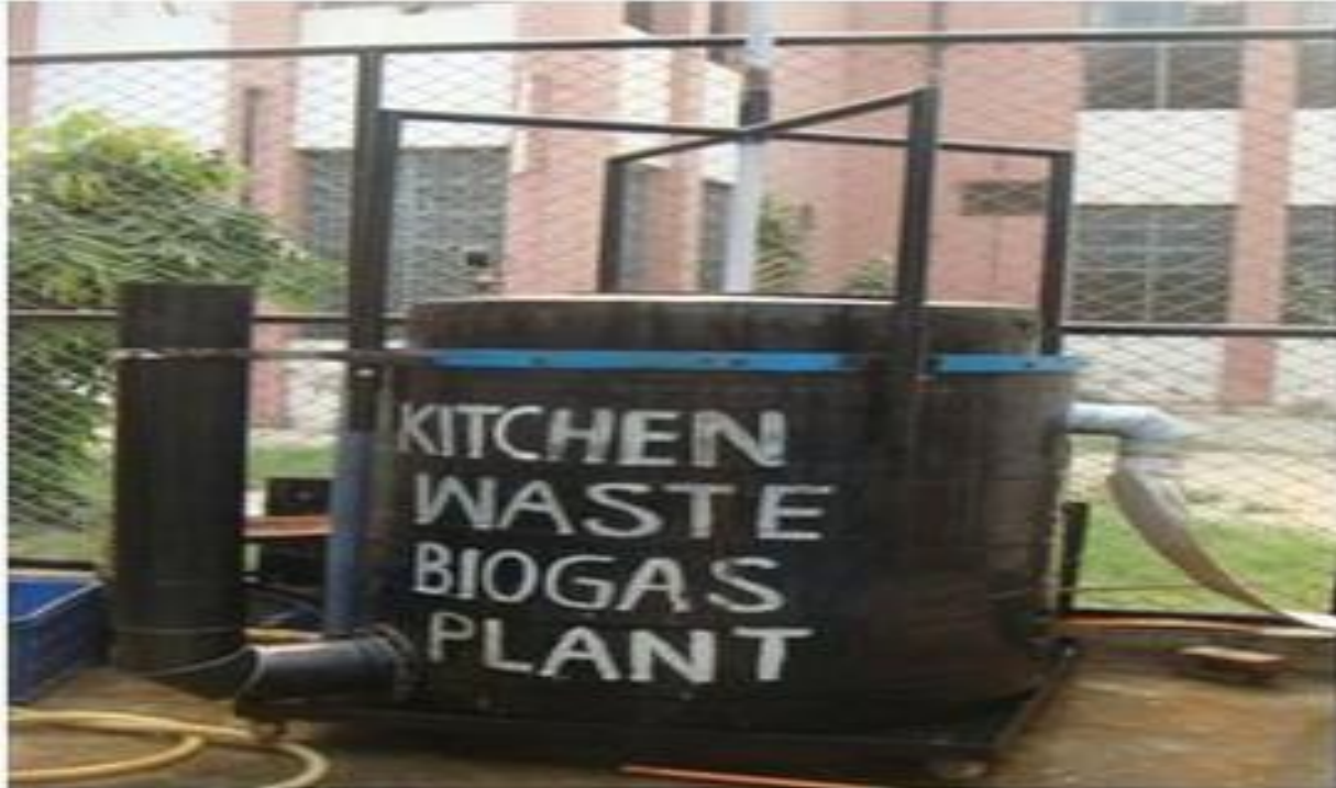
Fig. 2.2 A kitchen Waste Biogas Plant[3]
